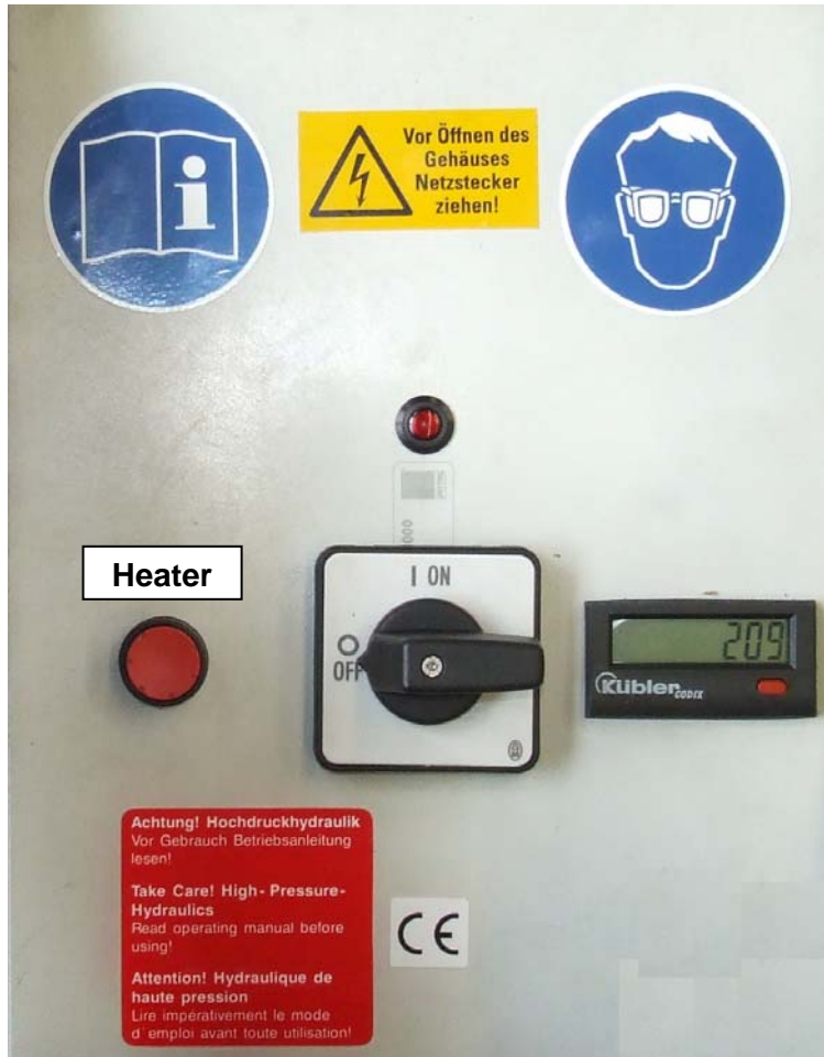
Fig. 3 Switch box, heater
